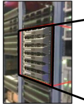
Google GGC Servers
